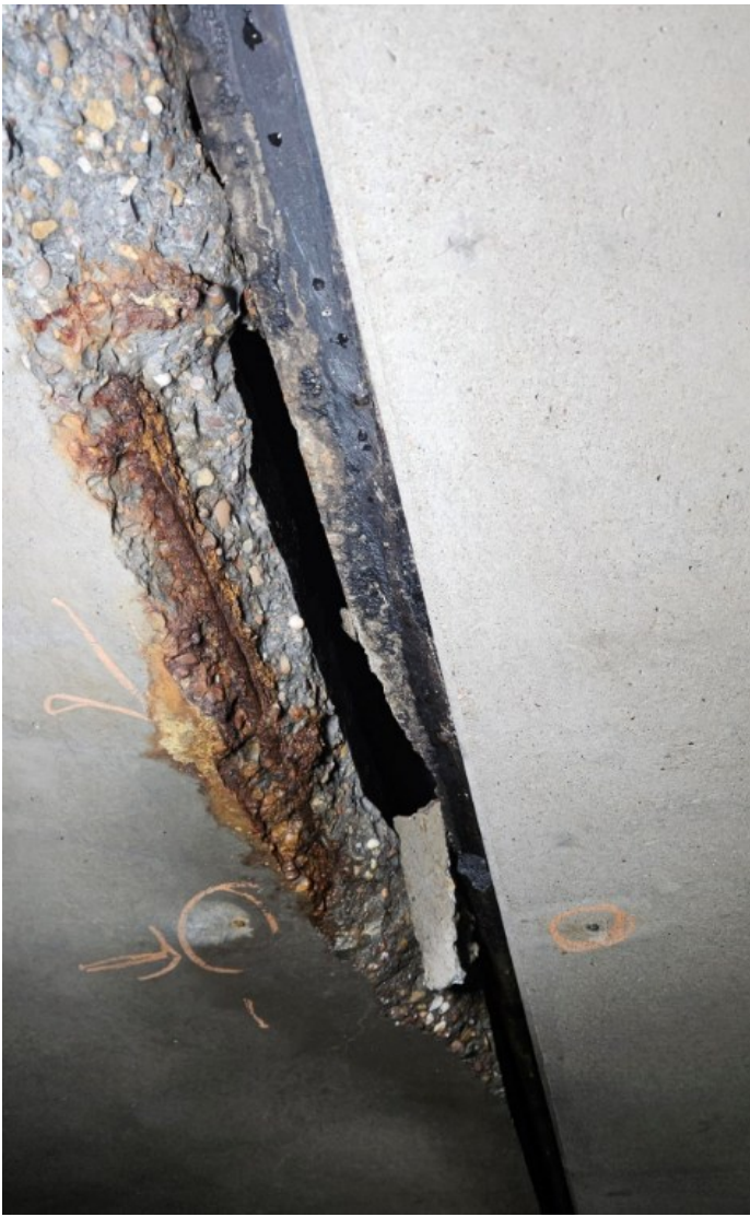
View of void above the culvert
